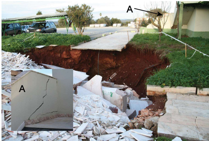
Figure 4. Karst cavity opened near a marble factory. This opening is probably related to a seismic event. This factory is located at point 4 in Figure 1.
