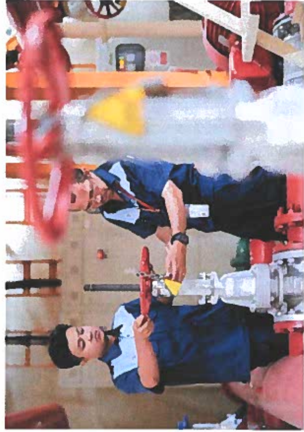
Above: Water treatment in PMI's Itabane, an affiliate Simpoena's manufacturing facility in Sukarejo
